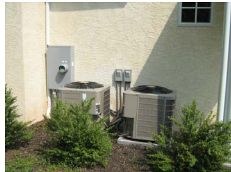
Air Conditioning Condenser Out of Level
