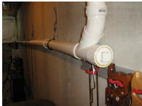
Improperly Sloping Waste Piping
