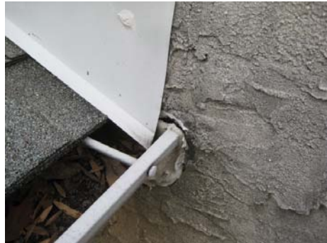
Hole in Flashing at Chimney
