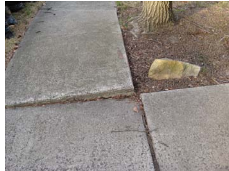
Trip Hazard (Front Walk)
