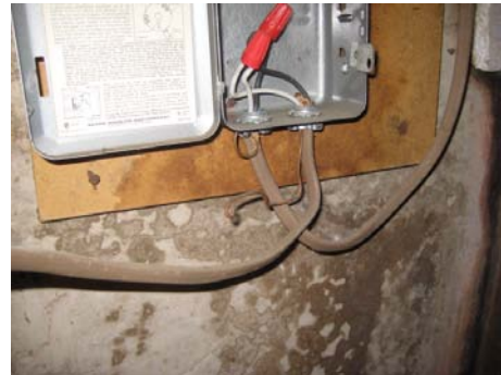
Ground Not Connected
