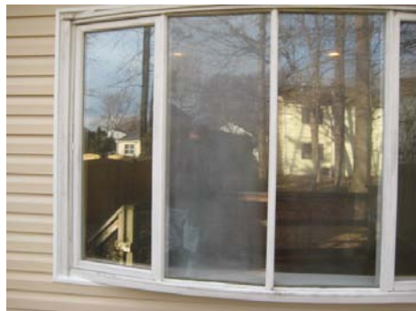
Broken Window Seal at Bay Window
