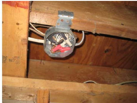
Open Junction Box
