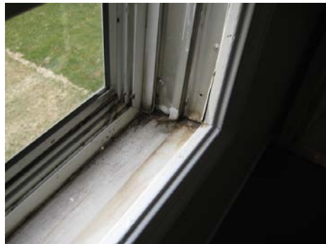
Rotted Sill in Master Bedroom
