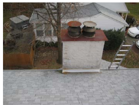
Rusted Chimney Cap
