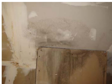
Water Leak in Garage from Chimney
